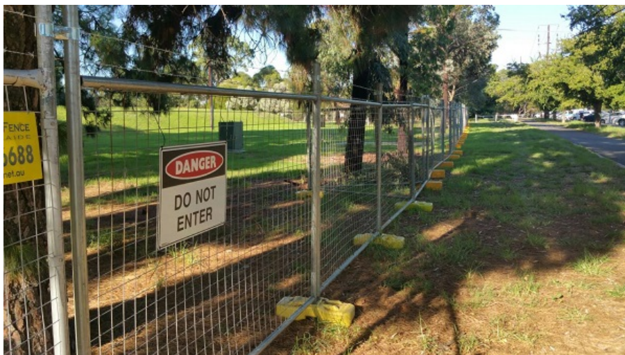
SA Water keeping you out of Kangatilla (Park 4) on the corner of O'Connell St and Barton Tce East (See the story 'Going Underground' in this e-Gazette)
