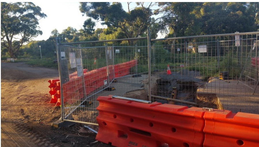
Part of Bonython Park (Park 27) just off Park Tce, taken over for sewer upgrade works
