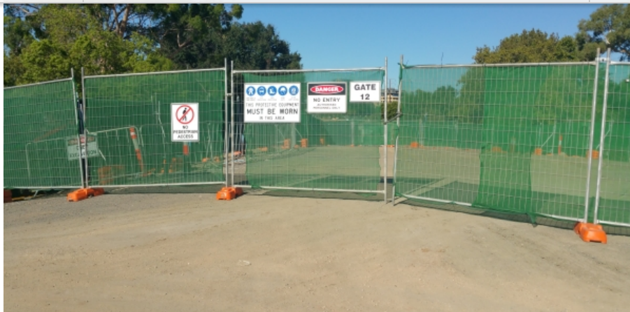
O-Bahn construction work preventing access to Rymill Park (Park 14) from East Tce
