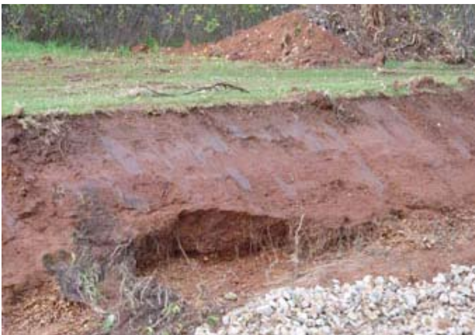
Left: Erosion resulting after just one heavy rain. Despite the rocks dumped in the 'creek' bed, erosion will go unchecked until the banks are revegetated fully—a process that could take five years according to one ACC source. Photo taken early May 2006 by Gunta Groves.
