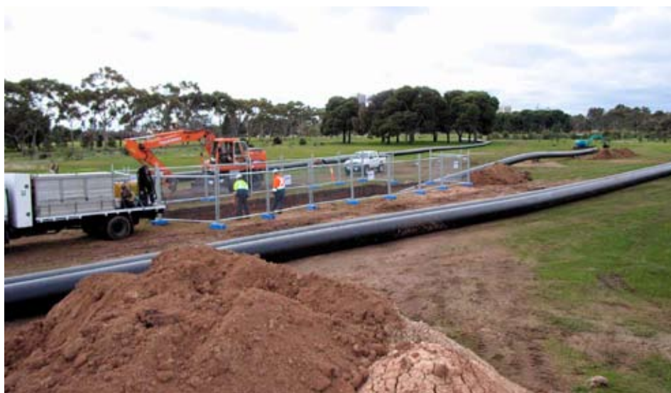
Above: Four lengths of 240m long pipes of 650mm diameter were deposited in the south Parklands in early June. Installation work finished at the end of July and some remediation continued into August.
