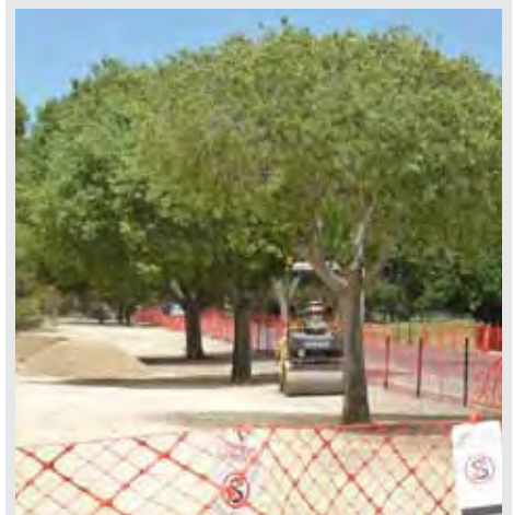
Below: Indecent haste of ACC car park construction works prior to survey without Tree and Critical Root Protection Zones, eastern side of War Memorial Drive adjacent North Adelaide Golf Course, looking south-east towards the City. Photos taken by K Henderson, 8 December 2012.
